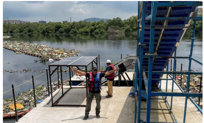
The unit intercepting floating plastic in the channel.
